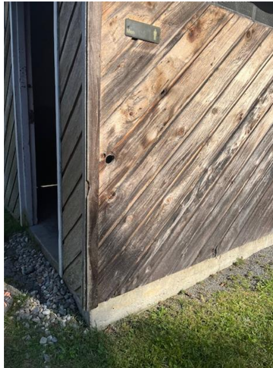
STEP INTO BUILDING NOT ADA ACCESSIBLE
