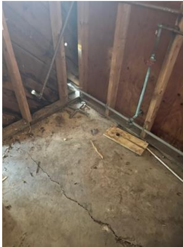
CONDITION OF SLAB
