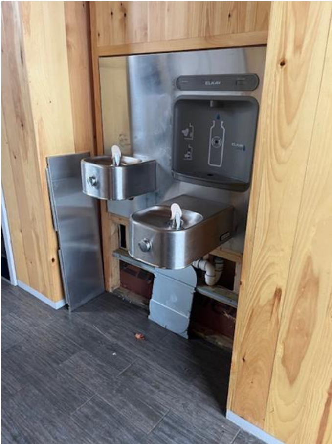
ACCESSIBLE WATER FILLING STATION
