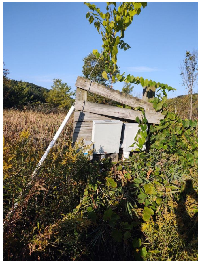
Pedestal / rink electrical panel & meter
