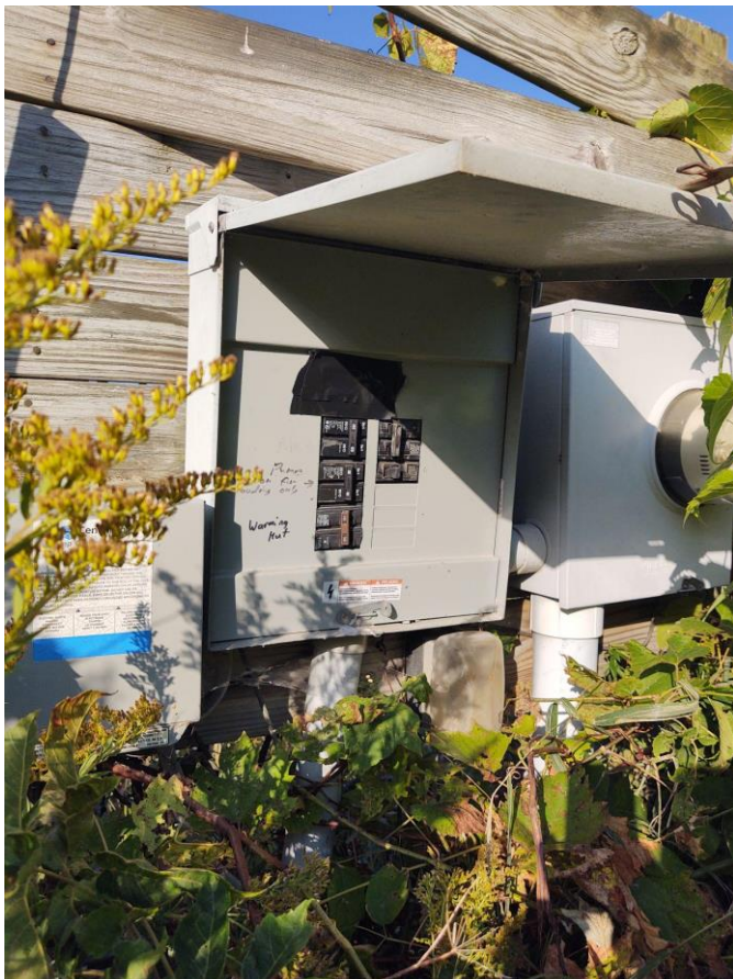
Rink electrical panel & meter
